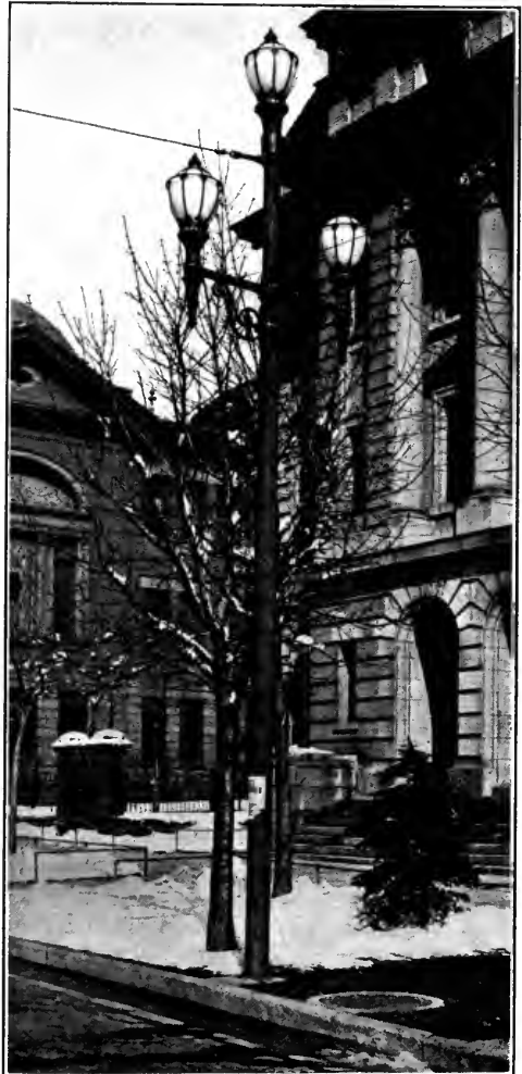
A COMBINATION LIGHT STANDARD AND TROLLEY-WIRE SUPPORT USED IN SALT LAKE CITY, UTAH
